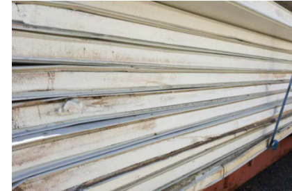
Wet panelling doesn't work
