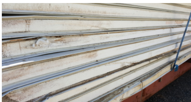
Figure 4. Room panelling materials that have become wet internally will not be effective insulators
