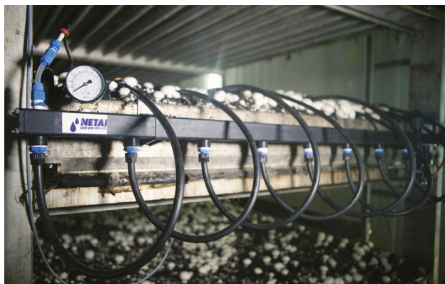
Figure 3. Netafim “ Mushroom Master ” irrigation system
