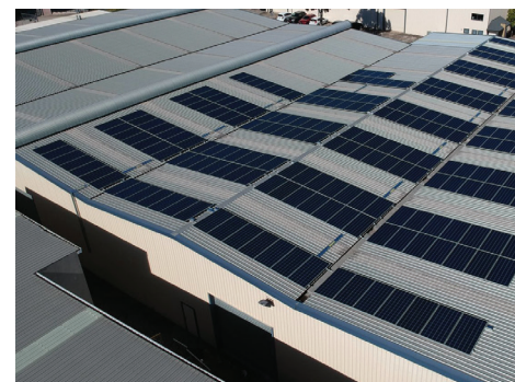
Figure 3. 100kW solar photovoltaic installed on a rooftop. Source: Spinifex Energy
